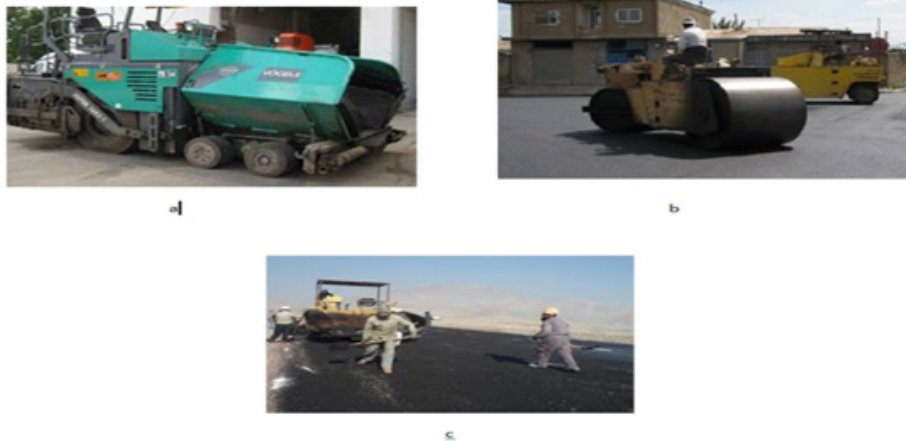
Figure 1 Process of asphalt work: a) finisher machine; b) rubber and steel rollers and c) shovelers
